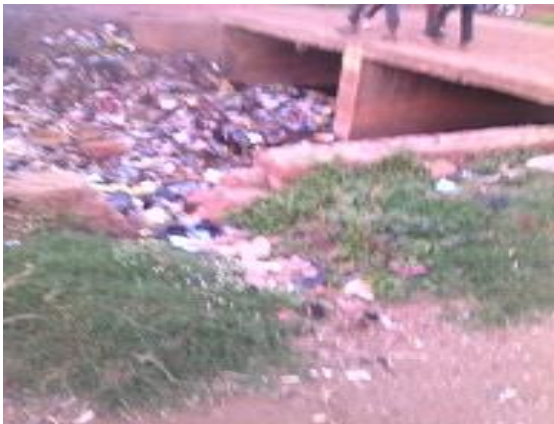
Fig. 2a: Culvert being destroyed by a gully in Wadata area.
