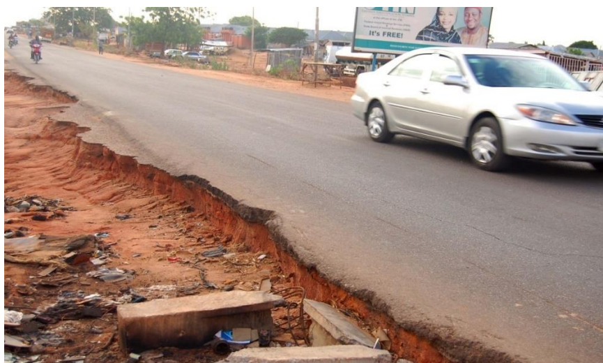
Plate 3: Cutting down of Bauchi-Gombe road by gully erosion
